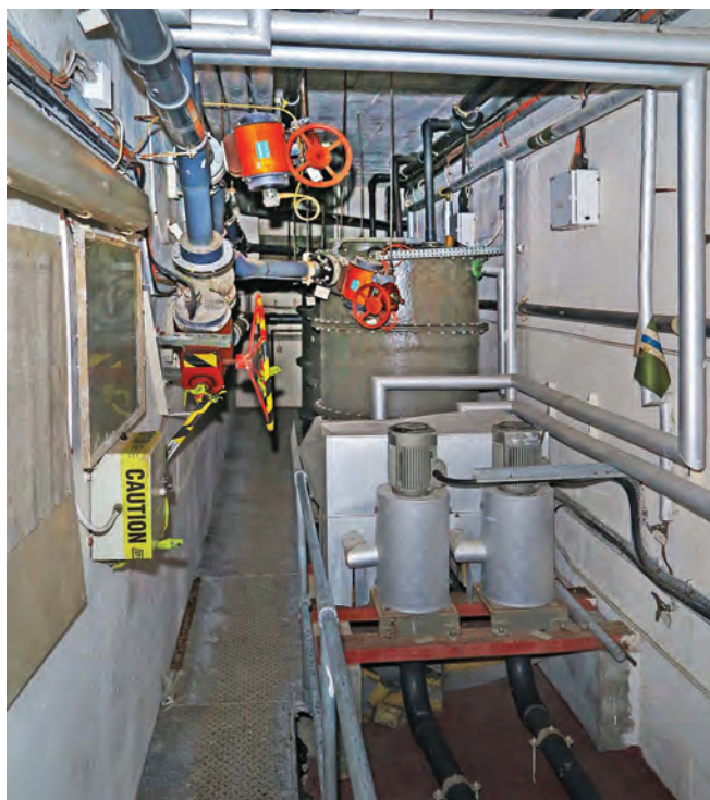
The air void between the inner and outer shell remained empty during WWII but in the 1980s refit it was a convenient space for all the new plant that was required. Photo Clive Penfold
